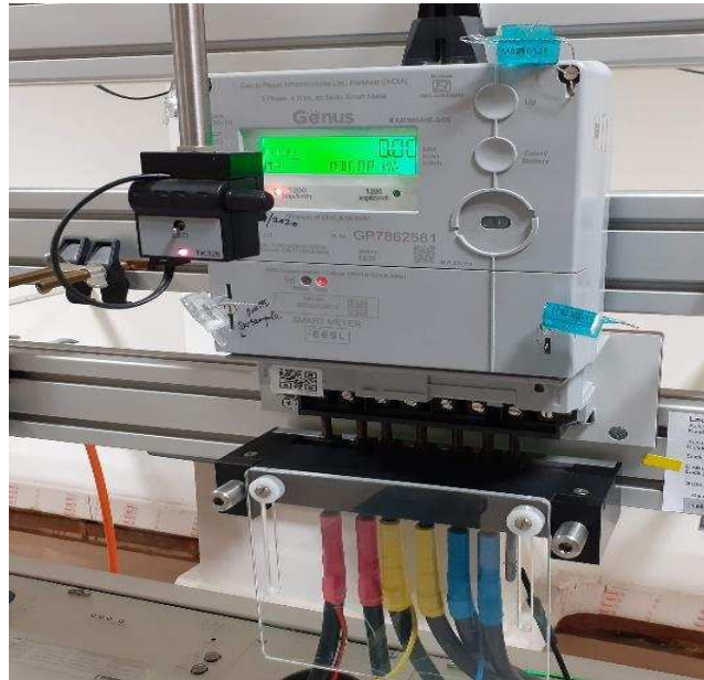
Testing of smart energy meter
