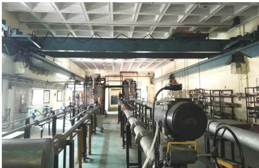
New 5 SS pipe lines along with associated instrumentations and controls of primary WFCF
