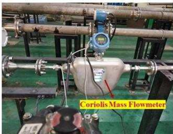
Installed artifact Coriolis mass flowmeter
